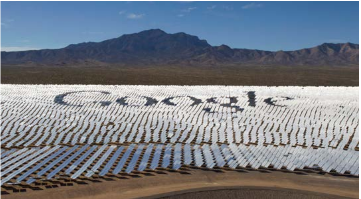
The Google logo is spelled out in heliostats (mirrors that track the sun and reflect the sunlight onto a central receiving point) during a tour of the Ivanpah Solar Electric Generating System in the Mojave Desert near the California-Nevada border February 13, 2014. The project, a partnership of NRG, BrightSource, Google and Bechtel, is the world's largest solar thermal facility and uses 347,000 sun-facing mirrors to produce 392 Megawatts of electricity, enough energy to power more than 140,000 homes. Credit: REUTERS/Steve Marcus
